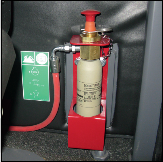
Fire suppression actuator in cabin/FS canopy LP is located close to door opening.
