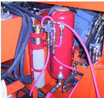
Ansul Fire suppression system
